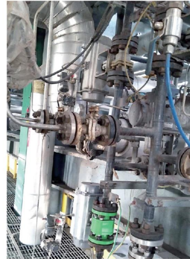
高压氮气 High-pressure Nitrogen
